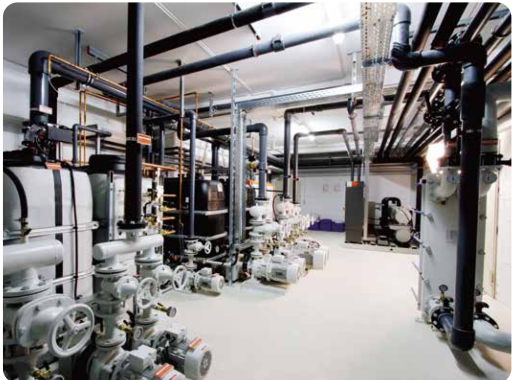
Central cooling plant with water treatment
