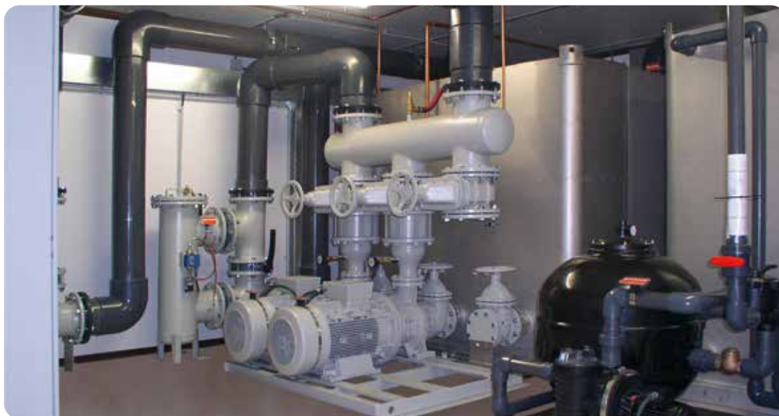
Containerised pump and tank group
