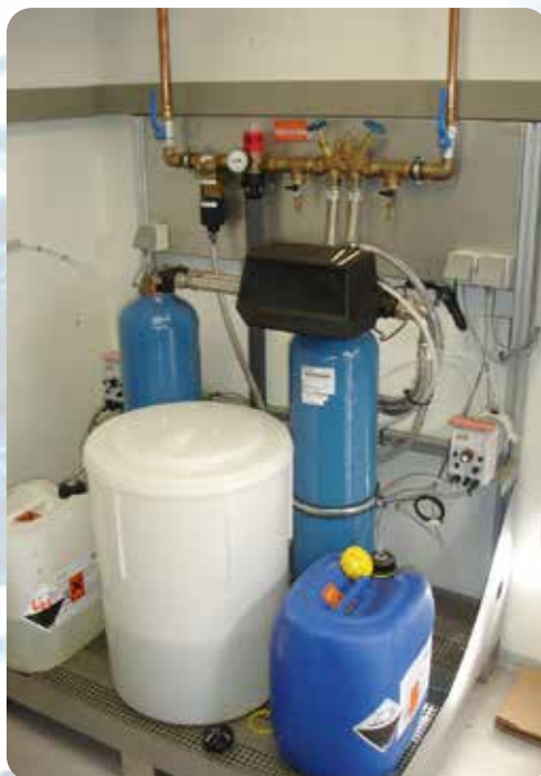
Double water softening unit to remove the minerals that form lime scale and dosing station for inhibitors to prevent corrosion, integrated into a container unit
