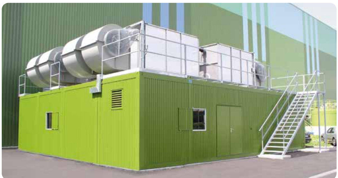
Containerised cooling plants are designed acc. to the individual demands
